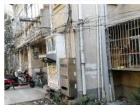
墙面立管破损、乱接✗
